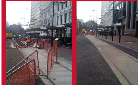
The first leg of the tram extension along Oxford Tce nearing completion
